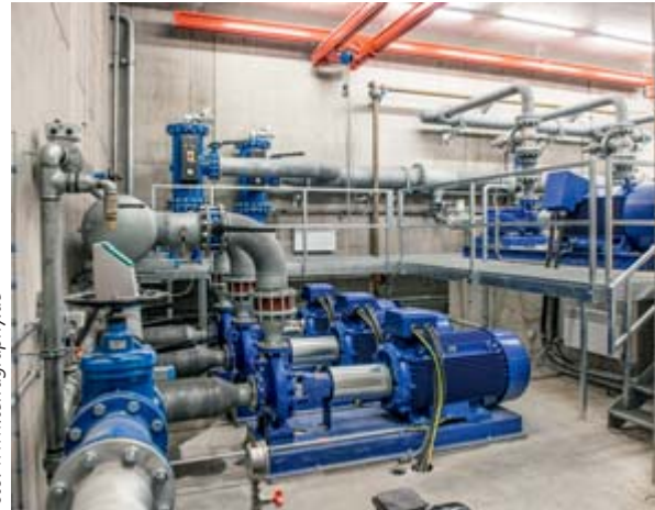
Blick in die Pumpstation Seebliga.
